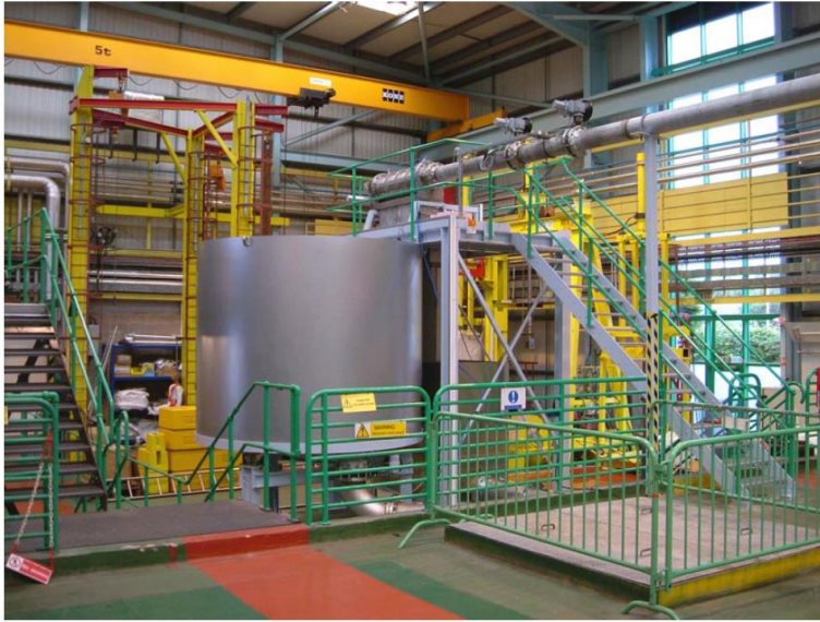
12-Tonne Weight-Tank System
